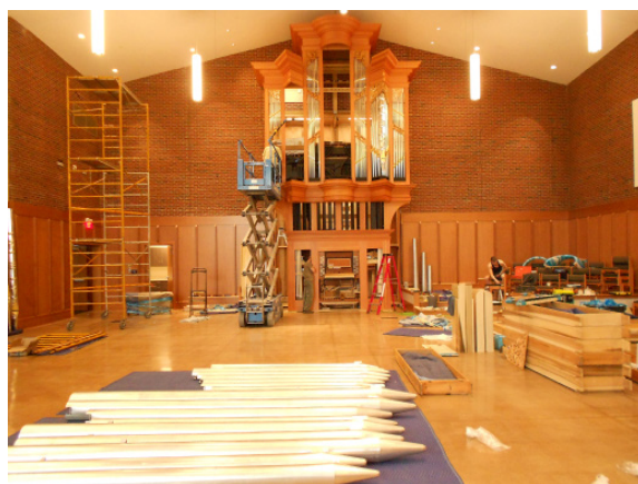
Installation in Lorain, May 3, 2019 Photo by Brian Wentzel
